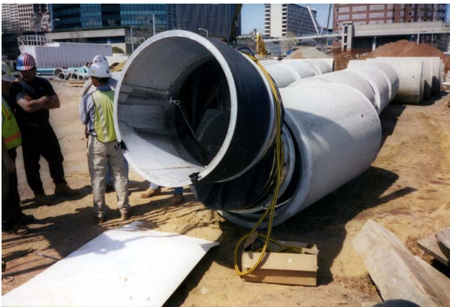
250-48 with a 42" bypass at a 22° angle
